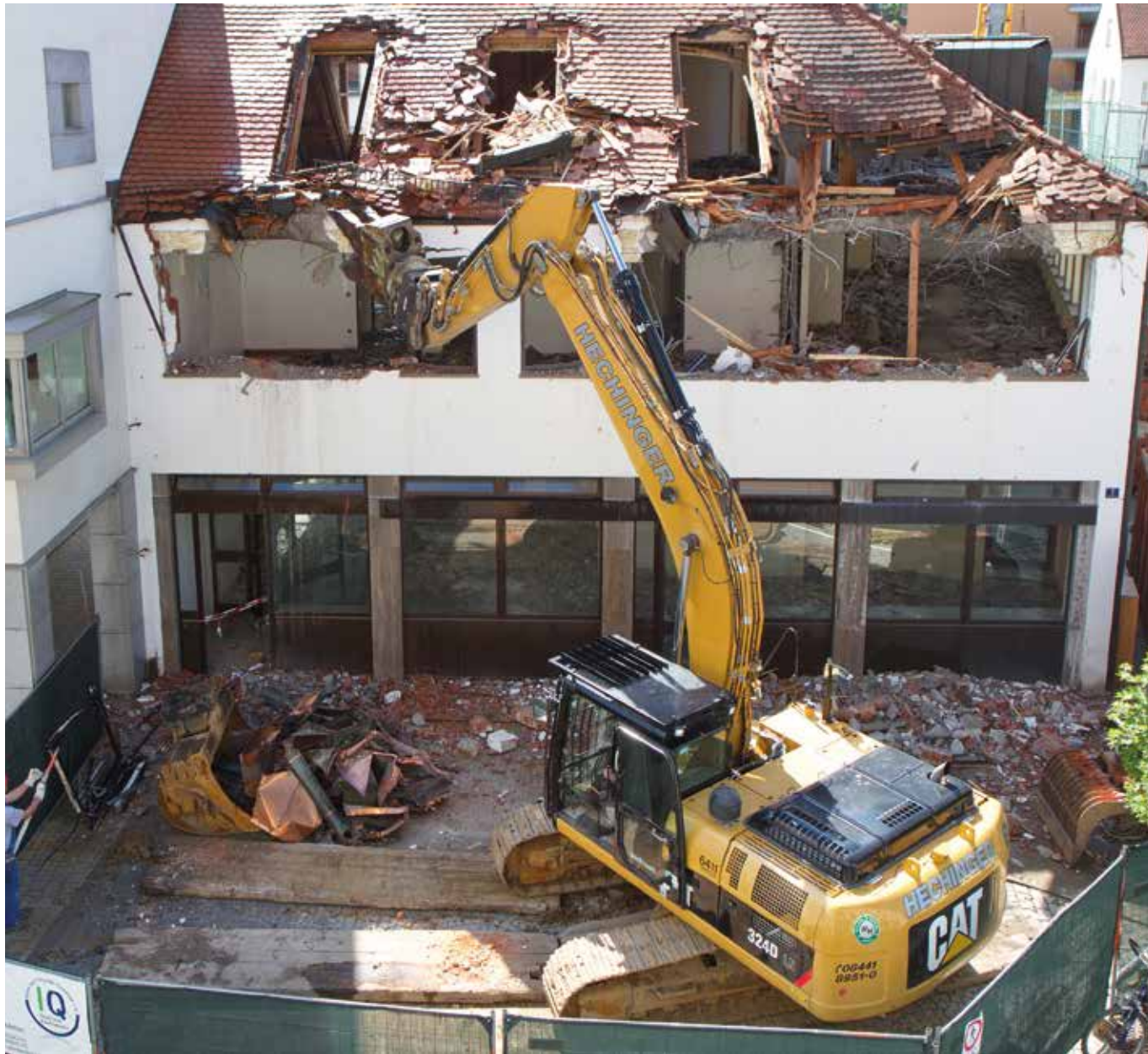
Demolition of buildings after only 10 - 15 years as an example of the waste of our resources. Art offers an incentive to enable the longer-term preservation of a building.
